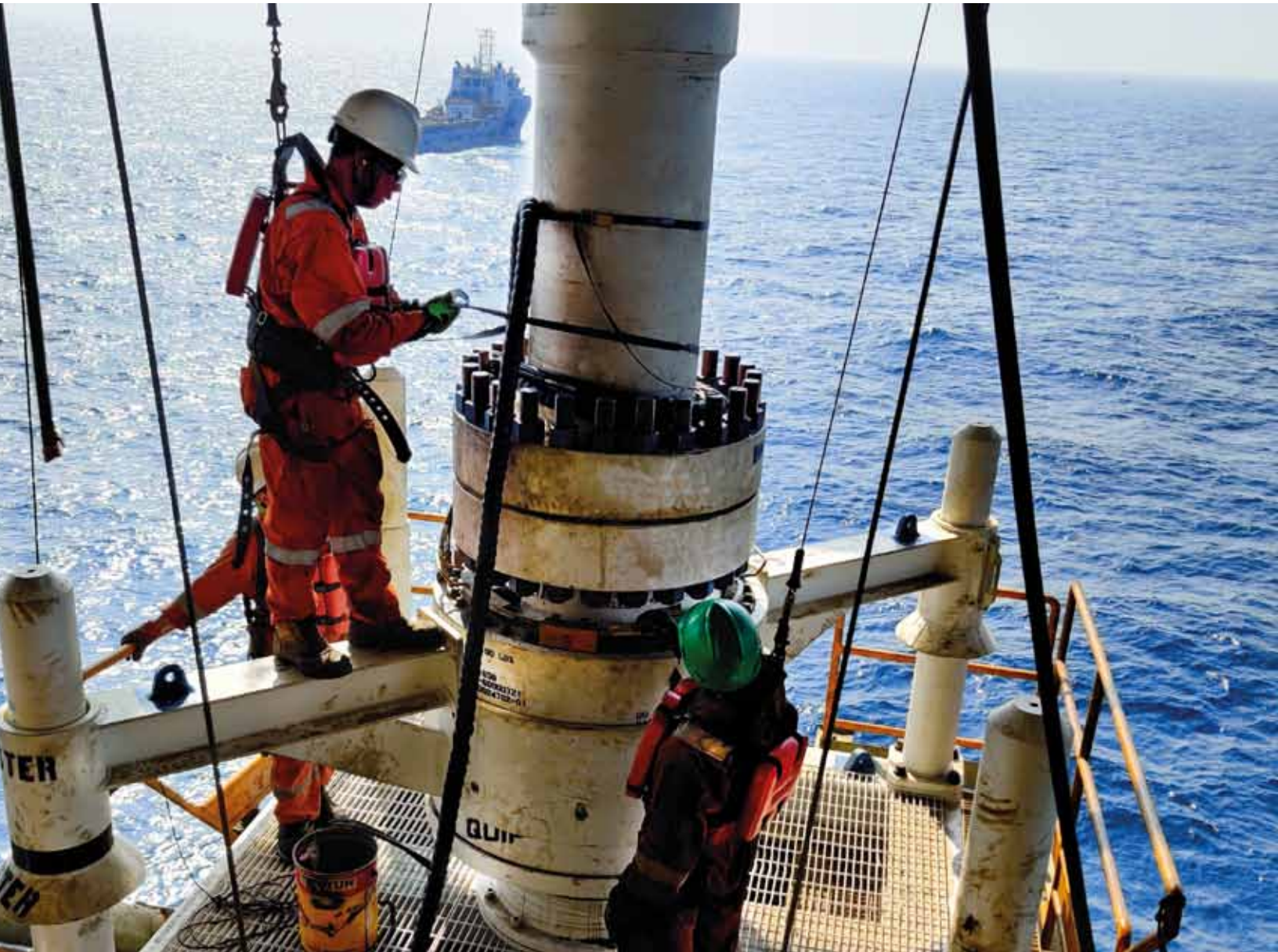
Subsea Wellhead during Drilling Campaign at B-80 Field, Mumbai Offshore
