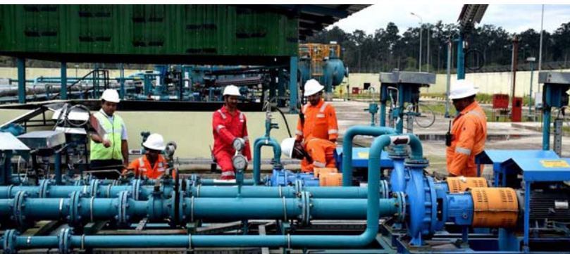
Operations at Hollong Modular Gas Processing Plant - Assam
